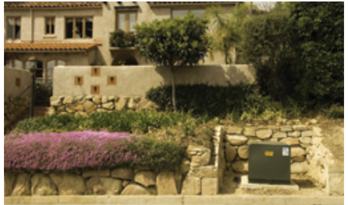
An aboveground transformer on lower Mission Ridge Road, similar to the one referenced below.
